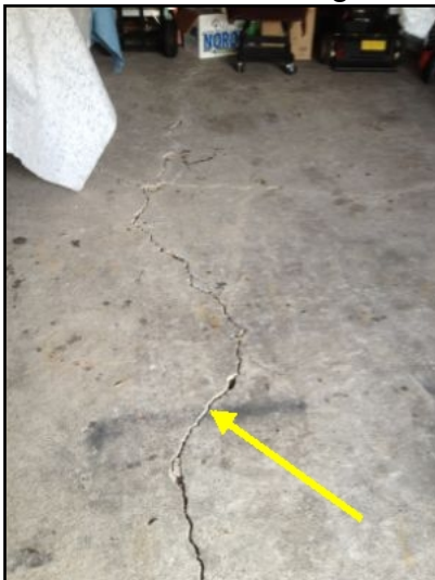
cracking in garage floor typical for it's age
