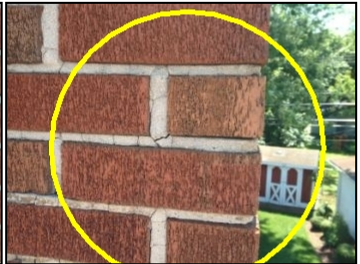
weathered mortar joints - tuck pointing needed
