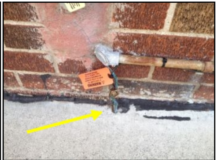
ground wire run through the cement driveway unsleeved
