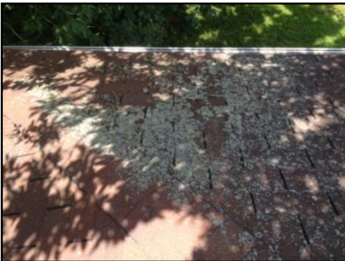
Garage roof beyond it's intended service life- OK at time of inspection
