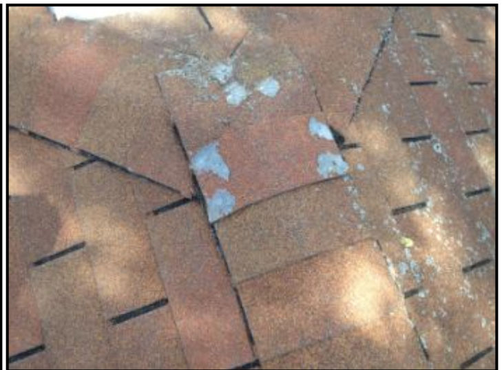
exposed nails in garage ridge cap shingle- seal to prevent water intrusion
