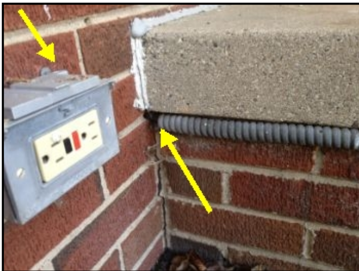
Broken GFI cover / exposed wires routed through brick wall
