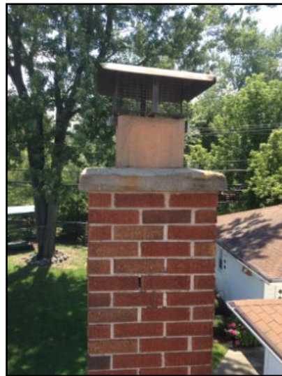
Roof Vent Caps
