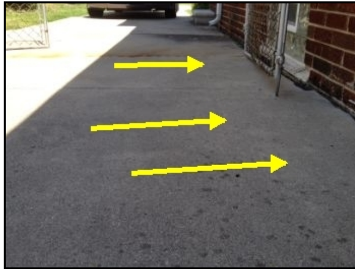
drive pitching wrong way toward house - possible water intrusion if left unrepaired
