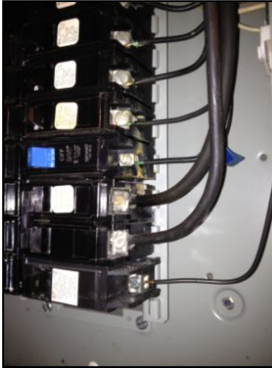
proper size aluminum service entrance cable
