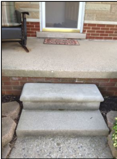
unequal step risers can be a tripping hazard @ front porch/entry
